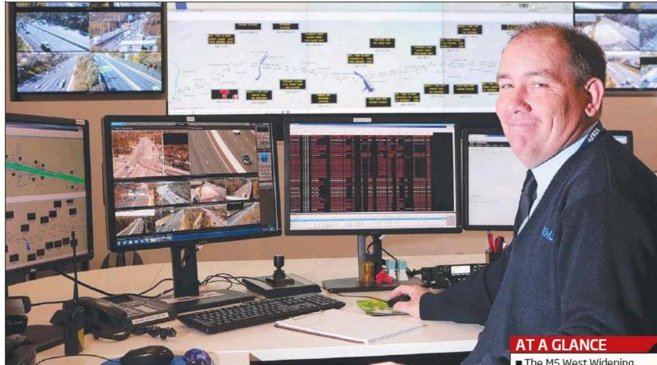
Senior M5 controller Stephen Tonlin at the M5 South-West Motorway Control Centre.
